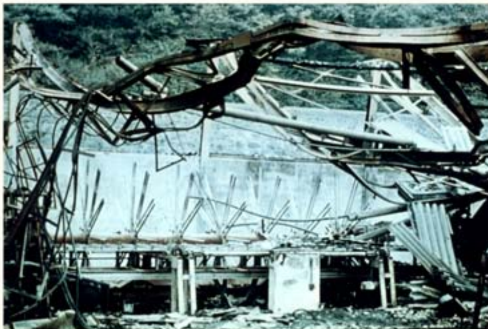
Part of a manufacturing plant after a dust explosion.
